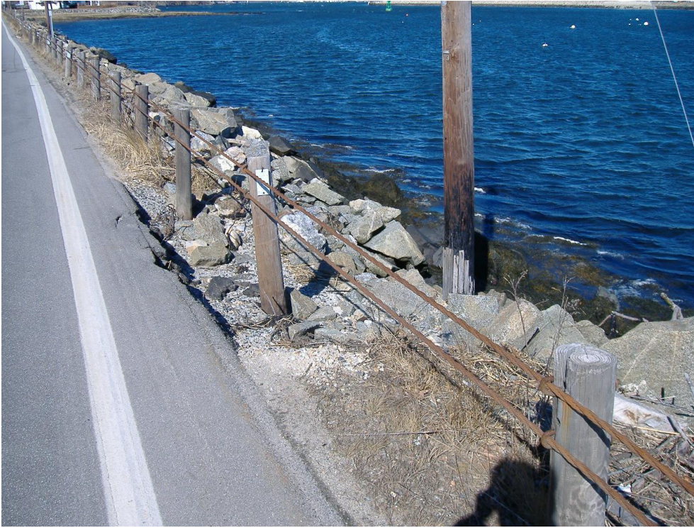
Figure 3: Causeway on Route 1B, Road surface erosion can be seen here and in other locations. This is caused by wind driven waves from the river-side of the causeway.
