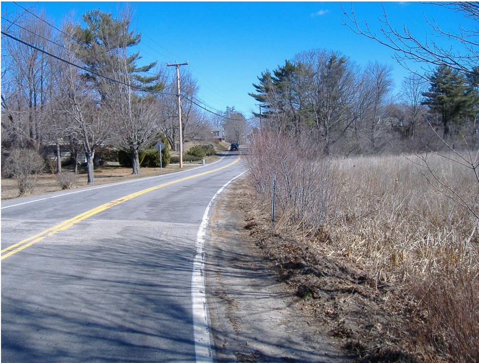
Figure 4: Route 1B near Pit Lane. Low section of road could be flooded and damaged during and storm surge event.
